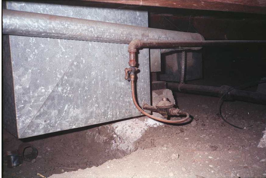
Photo 4 – Non-Safety Pilot system – Also note Condensation on Soils below Draft Hood
