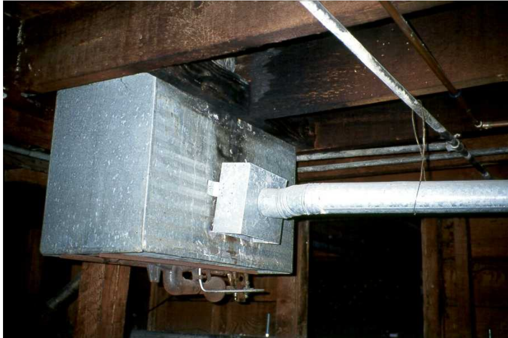
Photo 2 - Loose Draft Hood and Charred Framing
