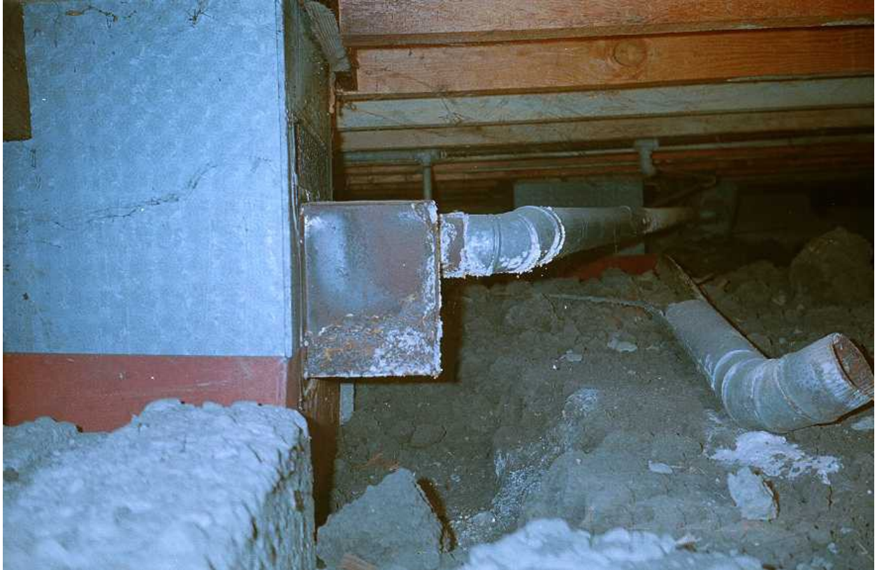
Photo 3 - Rusted Draft Hood and Discarded Old Vent
