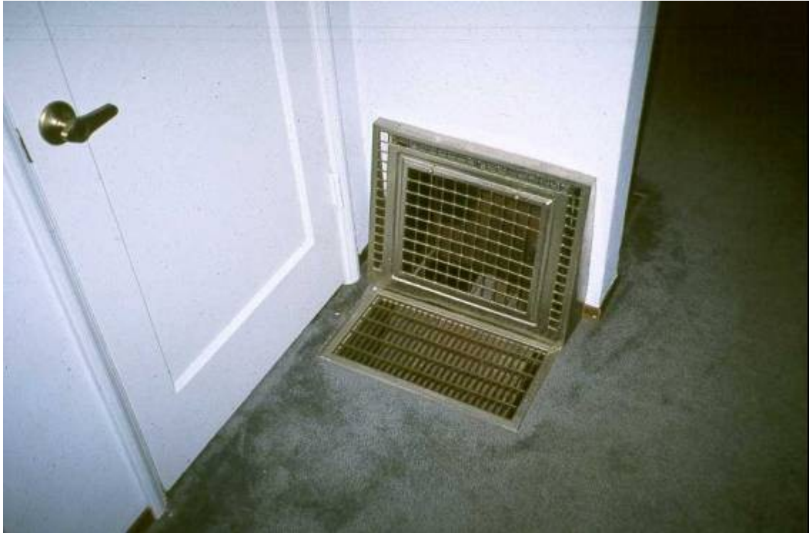
Photo 1 – Floor furnace next to door and within 6 inches of a corner
