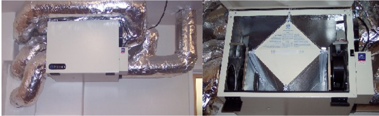
Fantech HRV Installed & With Access Cover Open – Photo Courtesy Douglas Hansen
